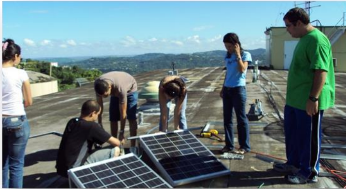
Students install solar panels to provide power for the OTG radar system in Mayagüez.
